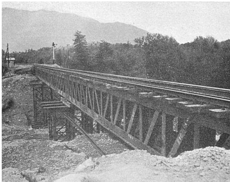
Figure 41. - Line 90. Bridge at Km. 75.92 between Ferentino and Morolo. Reconstruction was carried out by 10 Railway Construction Company, R.E. under Job N°. 90/69 from 8 June, 1944 to 30 June, 1944. The repair involved 3 Deck type U.C.R.Bs.
