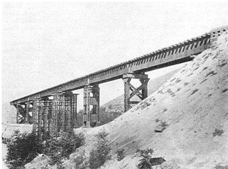
Figure 38. - Line 90. The Peccia Viaduct as reconstructed by N o . 1 Railway Bridging Section, R.E., under Job N o . 90/46, from 24 April, 1944 to 10 June, 1944. 46 Mech. Equip. (Tn) Platoon, R.E. carried out the earthworks. Crane girders from a steel works in Naples were used to span the gap.
