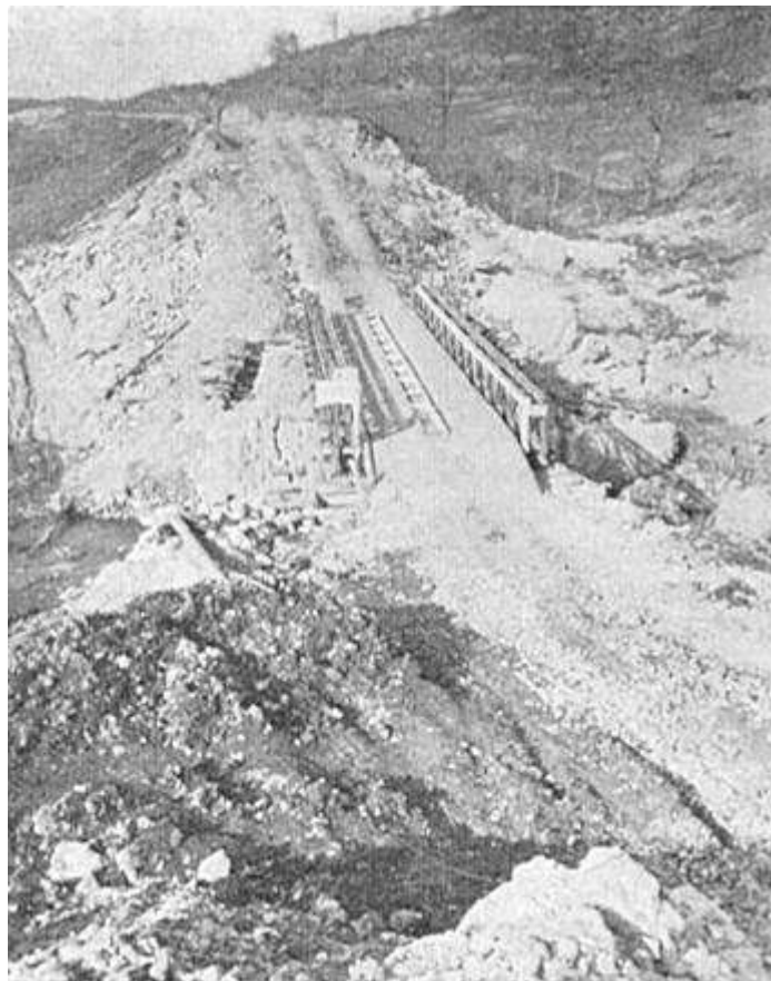
Figure 36. - Line 90. The Peccia viaduct approximately 1 mile North of Mignano, showing the complete obliteration of this 5 span viaduct. A Bailey Road Bridge was erected at a low level to take "Speedy Highway" over the Peccia stream.
